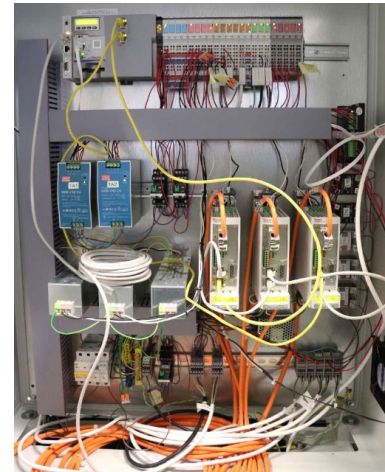
Figure 2: Control cabinet of the PLC
